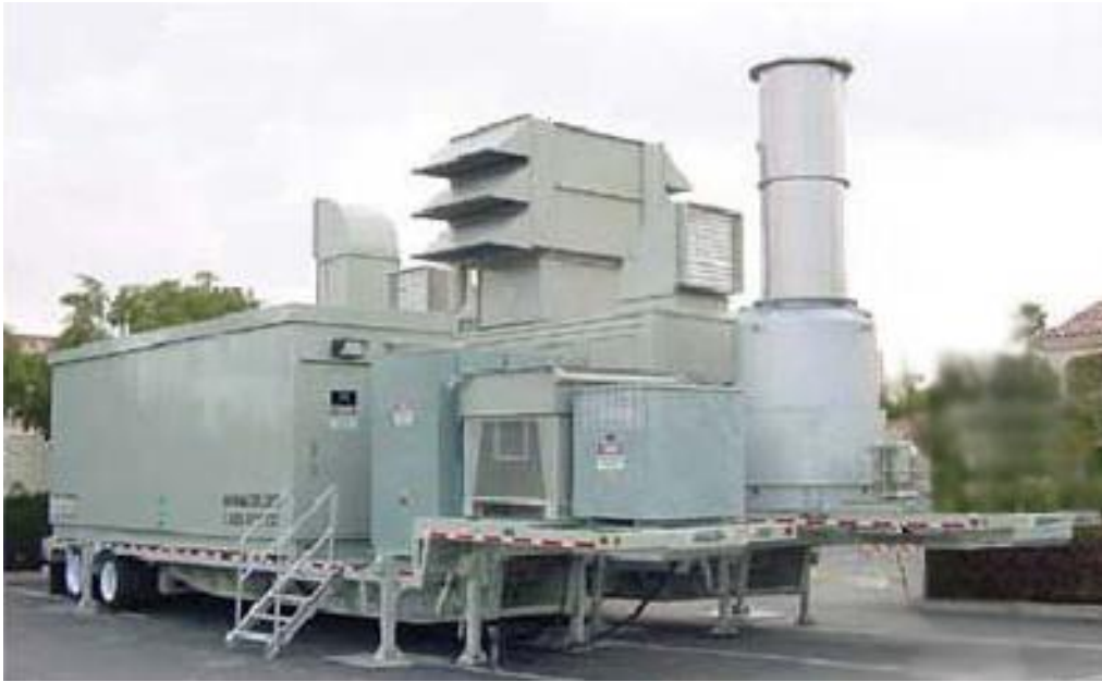
Taurus 60 Turbine Generator Set
